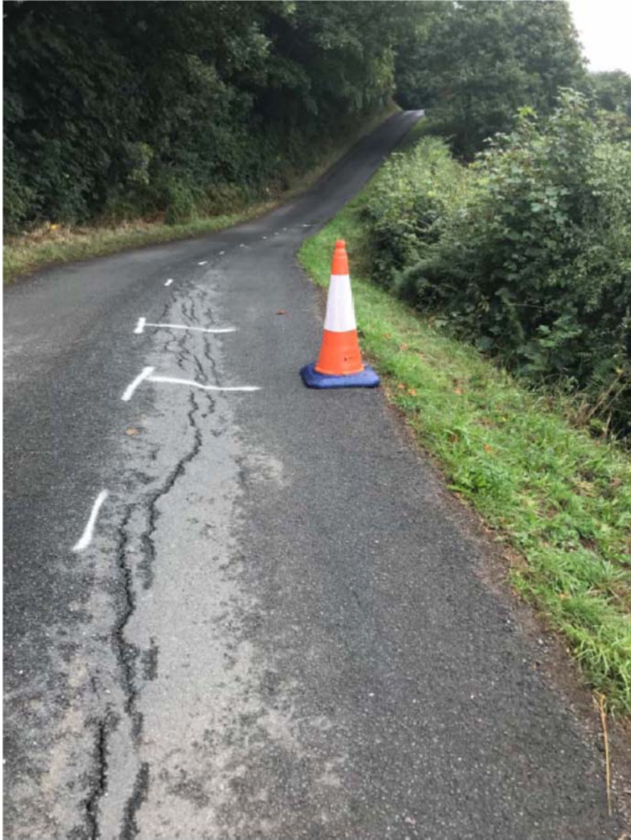
Egton Road, Aislaby Landslip;
